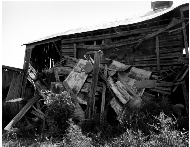
Figure 15 McCoy's log house/fort within damaged circa 1900 frame barn.
