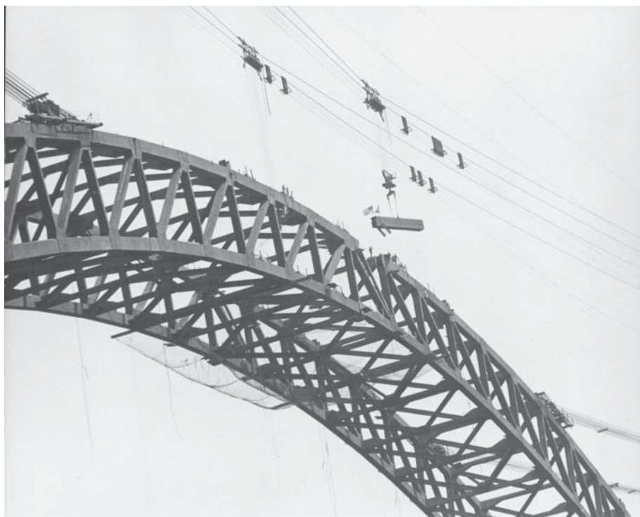
Final pieces come together for the arch of the New River Gorge Bridge
